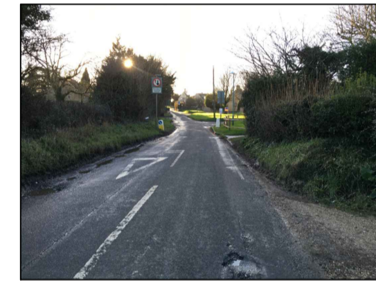
Narrow carriageway (<5m) could encourage vehicles/farm vehicles to overrun a new footway, double kerb option to be explored.
