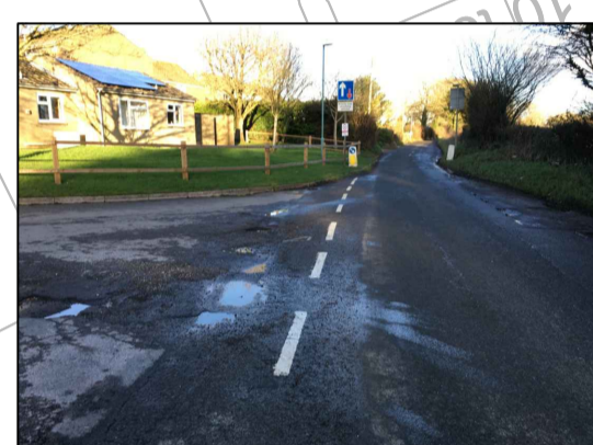
Land purchase required. Investigation into the exact extents of property, fence thought to be within highway extents
