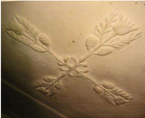
Part of the ceiling in Bell Court
